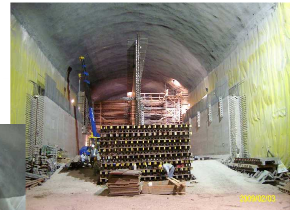
Construction of service reservoir structure in rock cavern 在岩洞內建造配水庫設施
