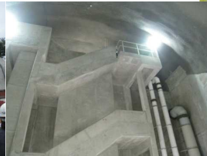
Completed service reservoir structure in rock cavern 岩洞內已完成的配水庫設施
